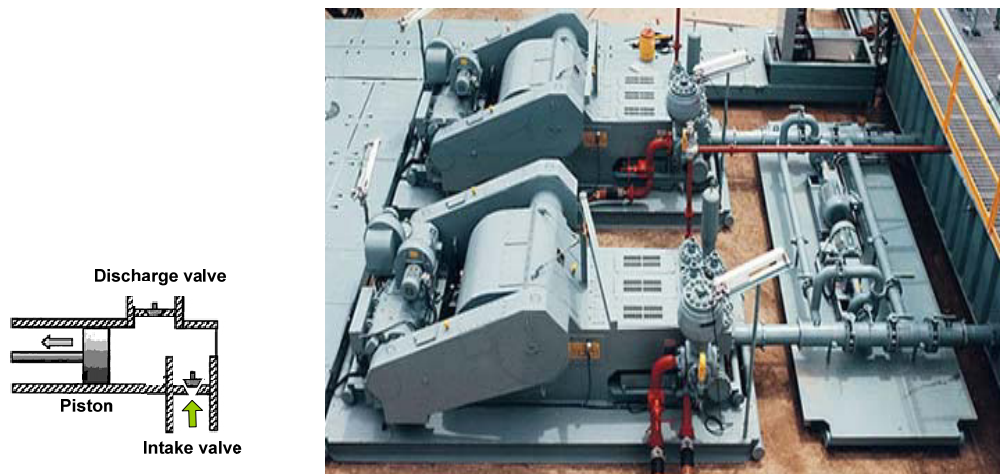
Figure 2-3: Two blue painted triplex (triplex means three pistons working in parallel), single acting piston pumps (single acting means acting only during on one of the two stroke directions). A single acting piston is shown to the left.
